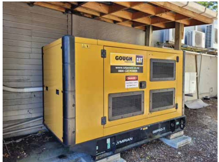
The large generator, with auto-start features, that keeps the vitals at Four Square on "life support", and, thankfully, the front door open.
